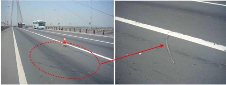
Fig. 11. Scratching on epoxy asphalt pavement on NSYRB.
