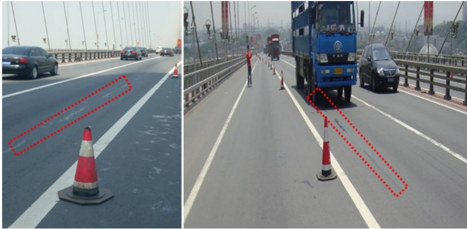
Fig. 3. Longitudinal regular cracks in the northbound drive lane on NSYRB.
