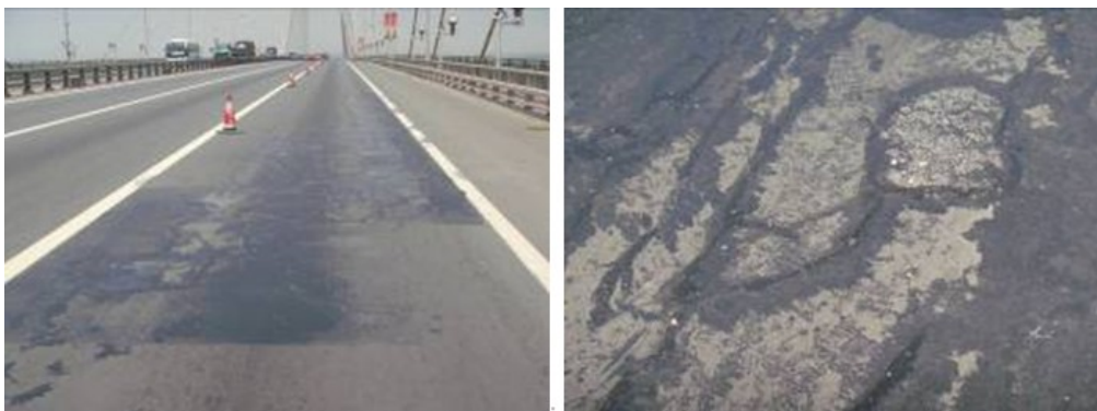
Fig. 7. Alligator cracks in the northbound slow lane on NSYRB.
