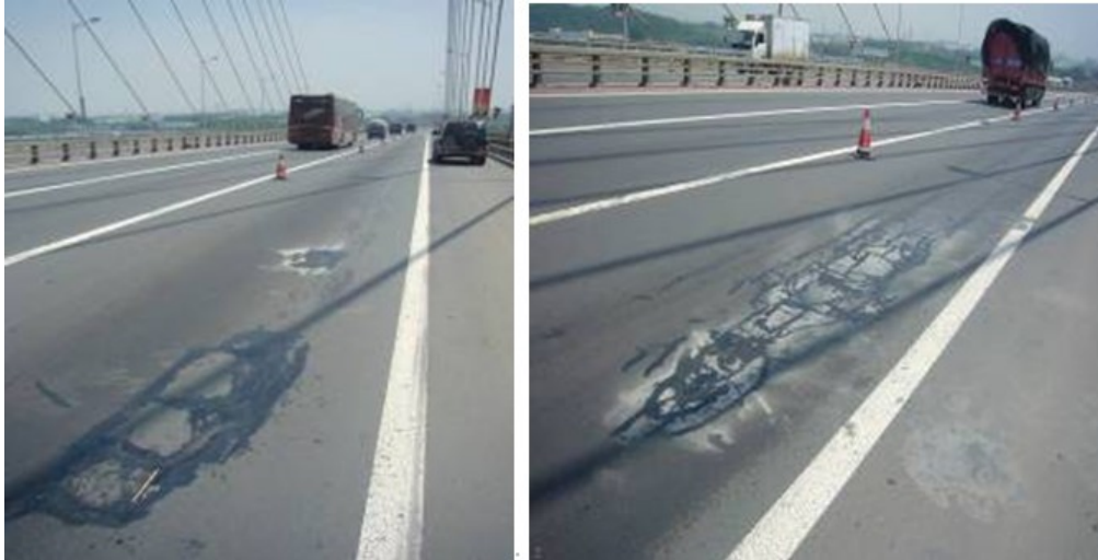
Fig. 8. Alligator cracks in the southbound slow lane on NSYRB.
