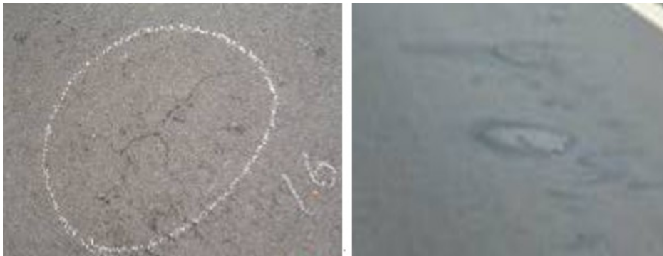
(a) Bubble crack
