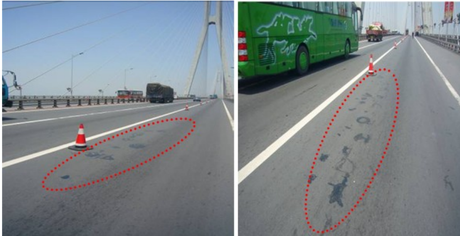
Fig. 5. Short hair cracks in the northbound slow lane on NSYRB.
